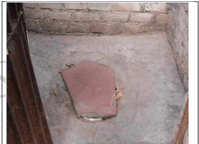
Figure-2: Photograph showing Toilet being used as bathroom (Dhar)
